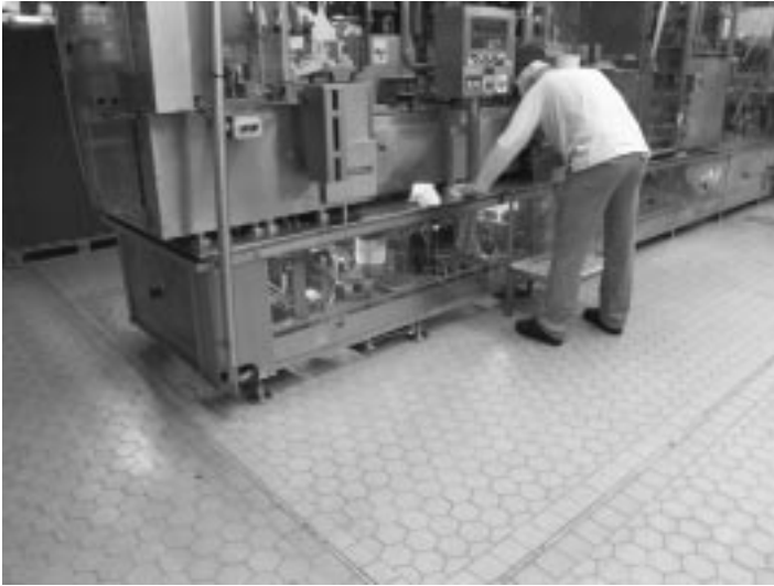
Fig. 15.6 Electrical equipment and valves below the machine in a visual and cleanable compartment 100 mm from the floor.
