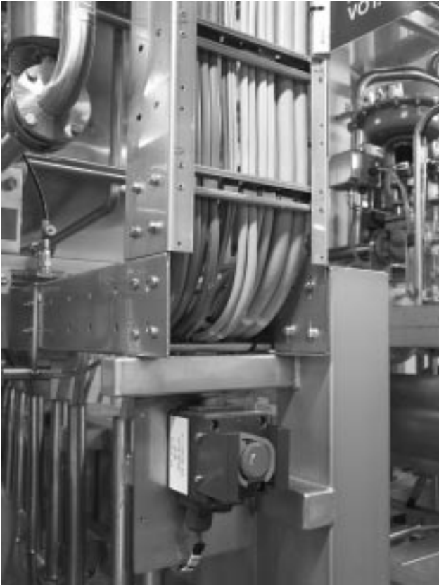
Fig. 15.3 Cables beside each other on a stainless steel cable ladder. Note the closed supports and cleanable conduits. Problem: the horizontal parts and omega rail of the cable ladder!
